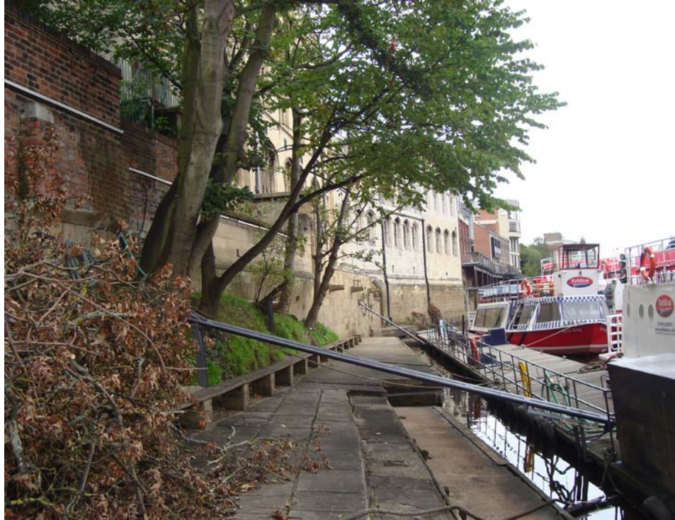
Views from the riverside by the York Boat Yard are restricted by tree growth. These trees have the potential to damage the fabric of the river wall and the location and appropriateness of these trees should be assessed
